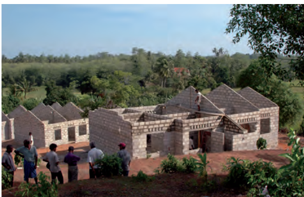
NA aid project Ape Gama (“Our Village”) in Sri Lanka: NA employees collected € 75,000 to help build a village for the victims of the tsunami in Sri Lanka. Dr. Werner Marnette, chairman of the Executive Board, promised to triple each euro donated. As a result, a total of € 225,000 was donated, which was used to provide new homes for many people.
